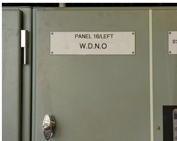
Figure 84 – Switchgear panel labelled WDNO
