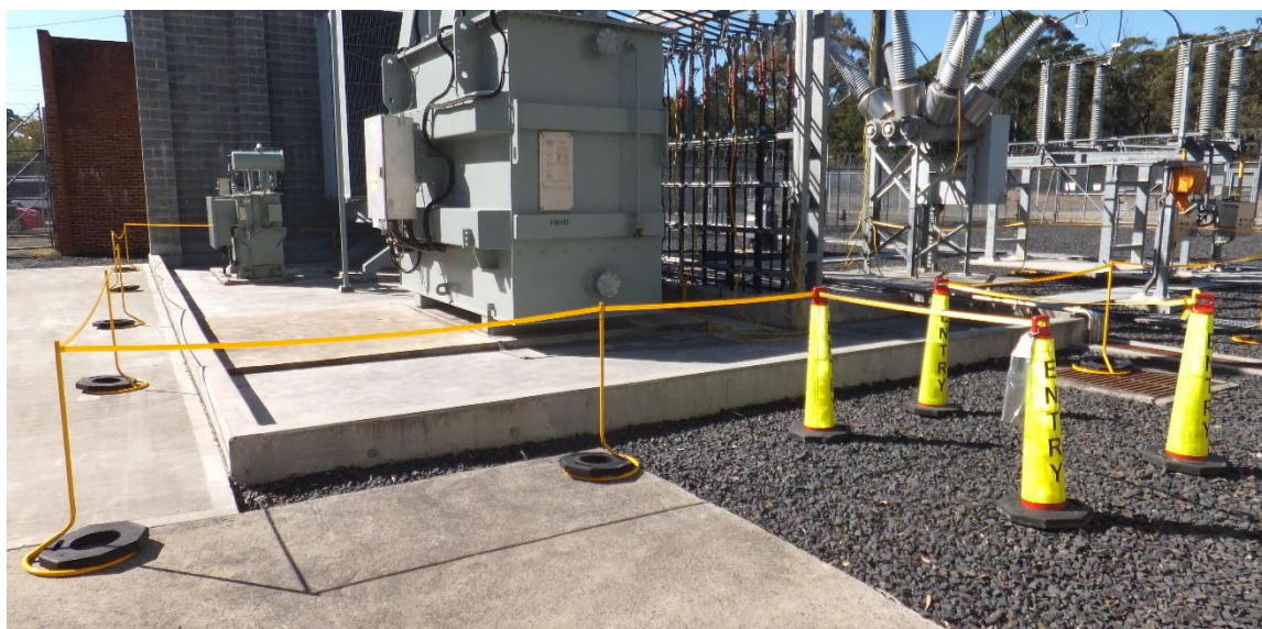
Figure 78 – An example of a safe work area defined by a yellow tape barrier.
