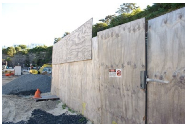
Figure 99 - Barrier to prevent workers encroaching minimum safe working distances
