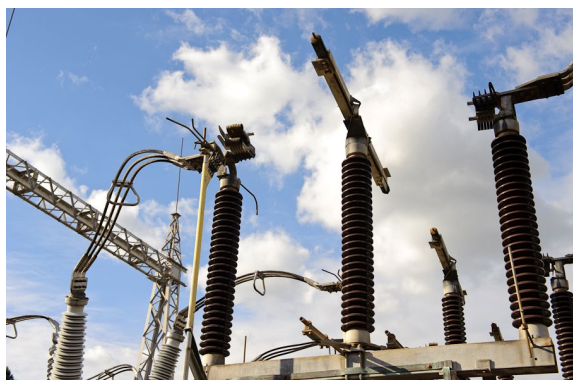
Figure 103 - Open 132kV isolator with closed earthing switch
