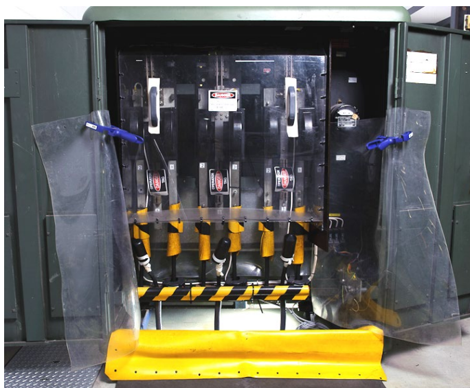
Figure 62 - LV temporary insulation and an insulating mat at a kiosk substation
