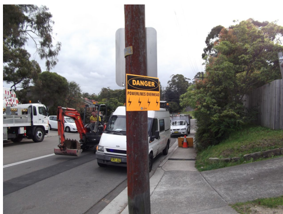
Figure 91 - Temporary 'Powerlines Overhead' warning sign
