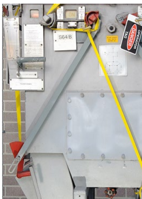
Figure 133 - Interlock engaged to prevent access to cable end box.
