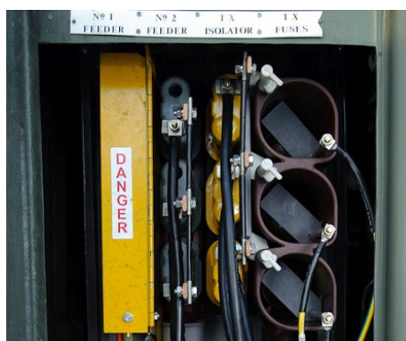
Figure 64 – An earthed screen in place covering live feeder spouts (note the busbar is earthed)
