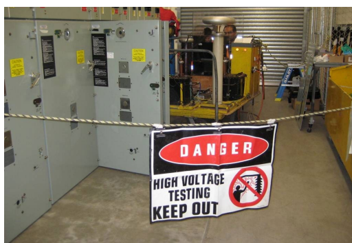
Figure 126 - Black and yellow rope barrier with danger notice
