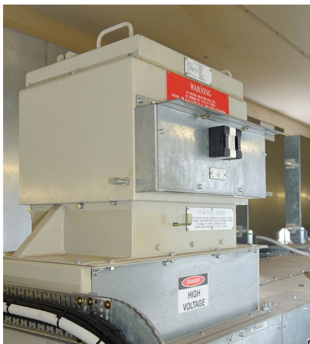
Figure 132 - 11kV—110V voltage transformer
