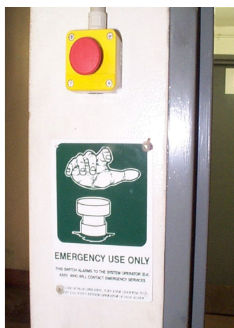
Figure 2 – An emergency switch in a Sydney CBD distribution substation
