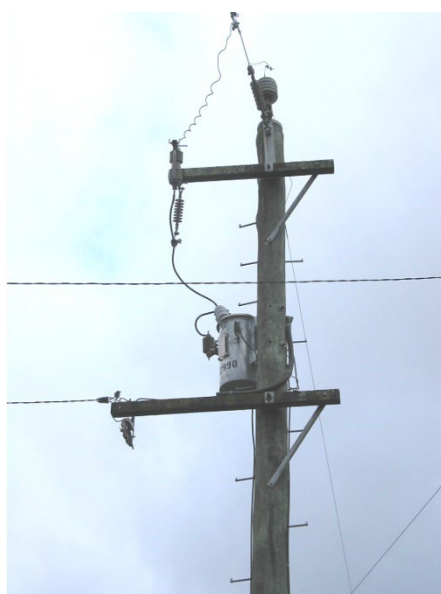
Figure 111 – A SWER substation
