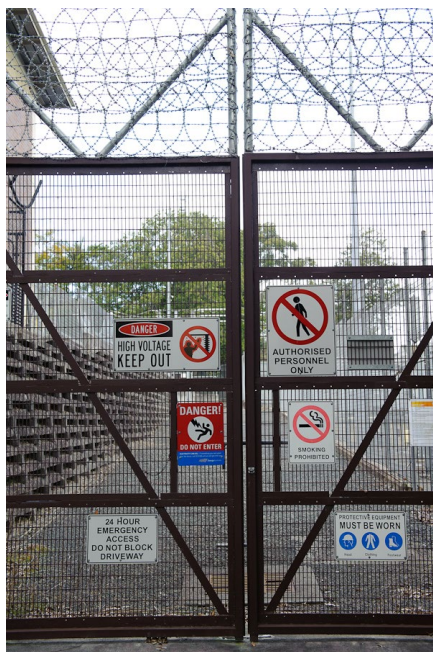
Figure 135 - Restricted access signs on gates at a substation
