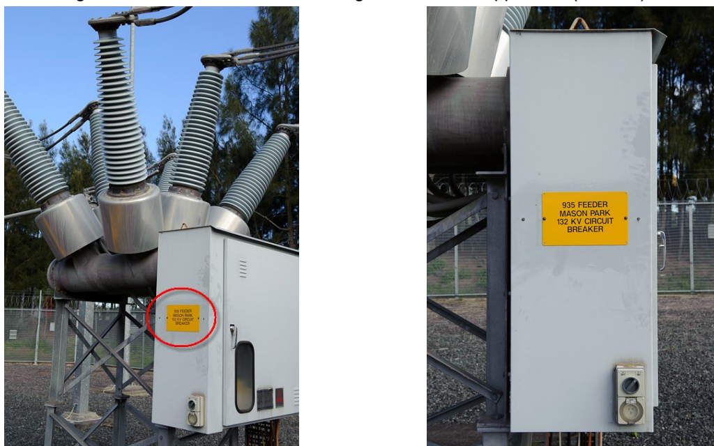
Figure 83 - Clear and permanent labelling on typical mains and apparatus
