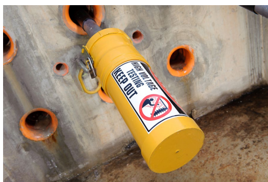
Figure 125 - Lockable cable termination with danger notice
