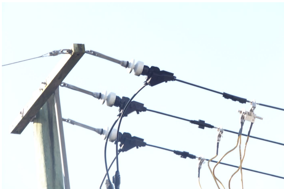
Figure 113 - CCT with earthing and short-circuiting equipment
