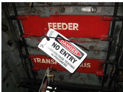
Figure 127 – HV testing tag applied
