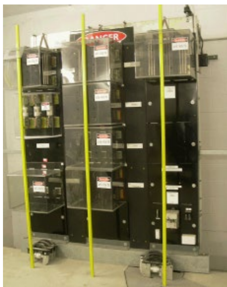
Figure 61 - A screen over exposed LV apparatus in a substation.
